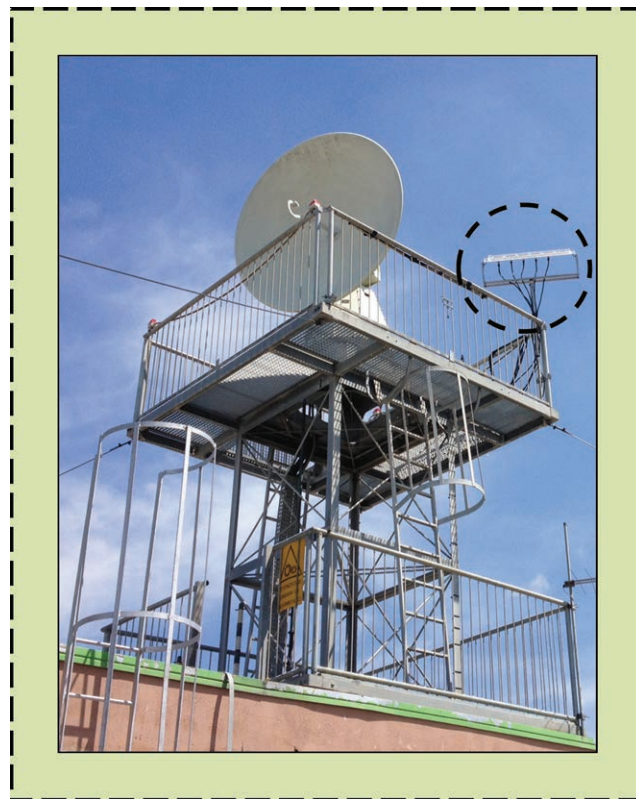
Figure 1. Photo of the antenna installation (shown in dashed circle).
