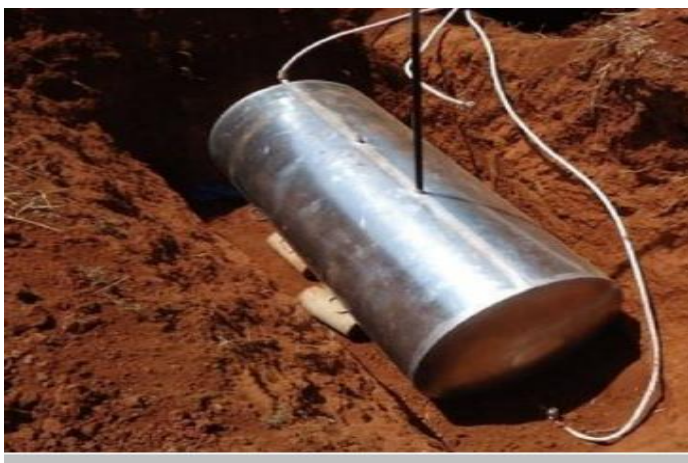
a- Underground tank
